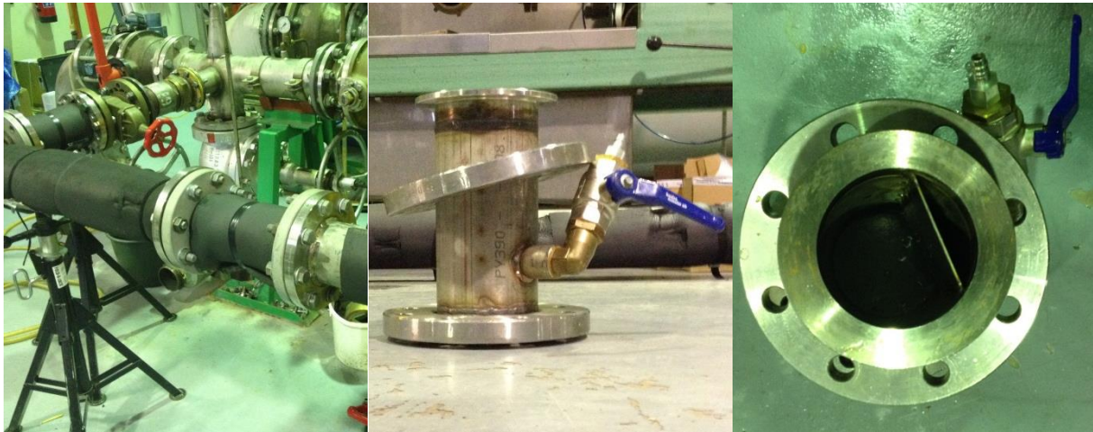
Figure 111 – Installation position (at the start of the measuring section) for the adapter with which the compressed air is blown into the pipeline
