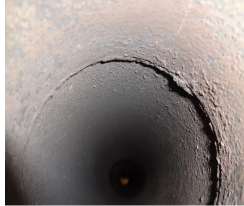
Fig 37. Downstream Meter Run
