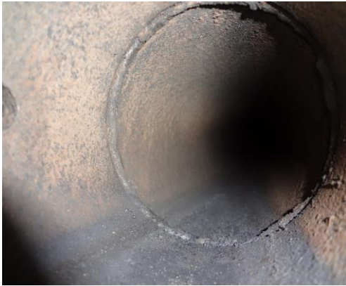
Fig 36. Upstream Meter Run
