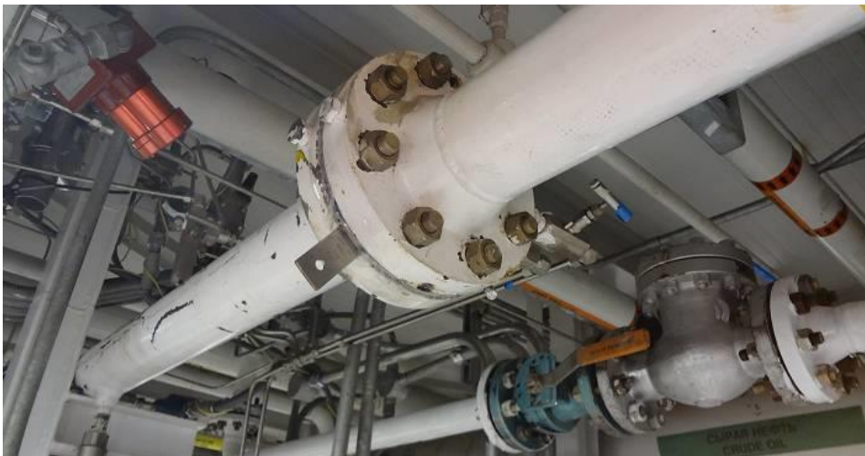
Fig 33. Polar Lights 4" Paddle Plate Orifice Meter with Diagnostics Installed.
